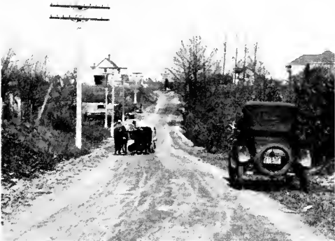
Example of early road construction under the "seven-year program" of 1908. Ox carts and flivvers share the improvements on an equal basis.
